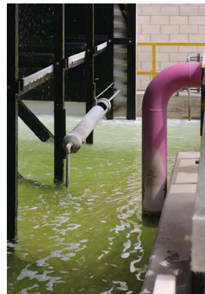
Reclaimed water used in the cooling system of the Malburg Generating Station
