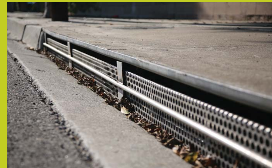
Stormwater catch basin screen
