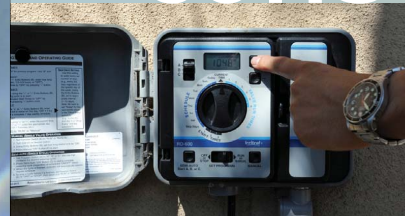
Energy-saving irrigation controls
