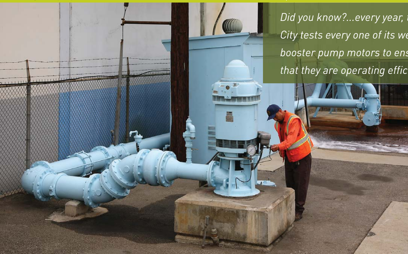
Testing water pumps to maintain maximum efficiency
